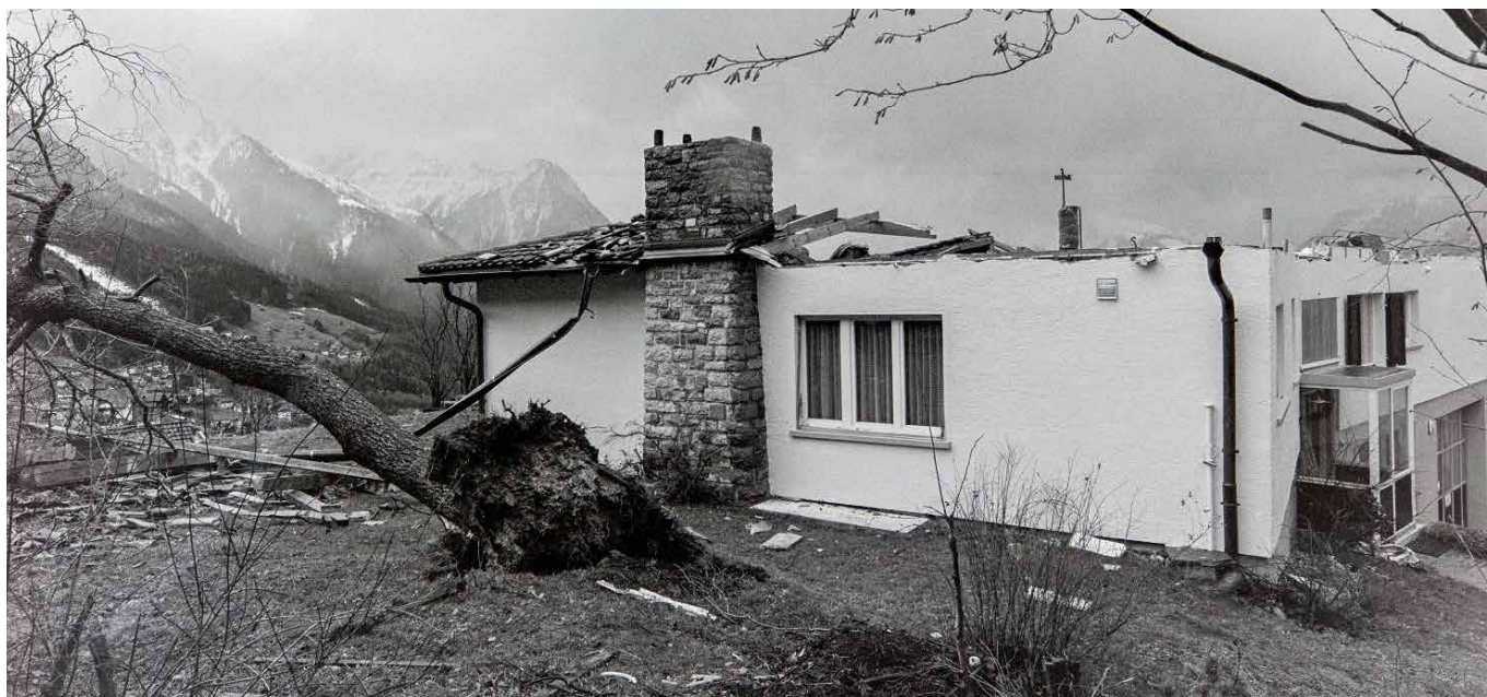
On 26 December 1999, Cyclone Lothar sweeps over Liechtenstein and leaves behind massive damage.
